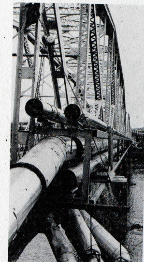
Pulp stock and white water pipelines installed on the International Bridge.
